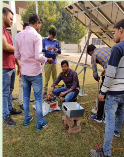
Training on Solar Plant Electrical Connection
