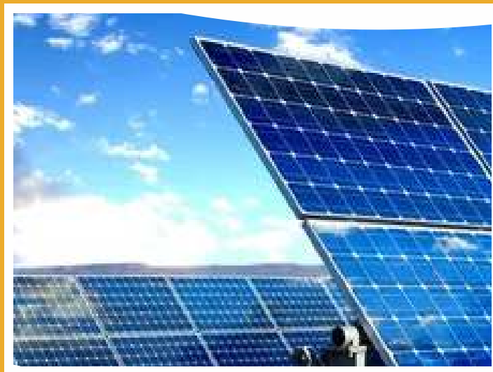
UP Solar Park-75 MW Parasan, Jalaun
